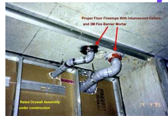
Northern Castles, North York (now Toronto), Ontario, Canada, April 1995: Set-up for subsequent code infraction in plastic pipe wall penetrations: Improper hole sizing. Firestops (in the walls) the plumber considered to be the drywaller's responsibility. Floor openings are properly done in this case, with intumescent pipe collars and firestop mortar. The intumescent will expand and choke off the melting pipes. Drywall mud does not work as a plastic pipe firestop in the wall.
